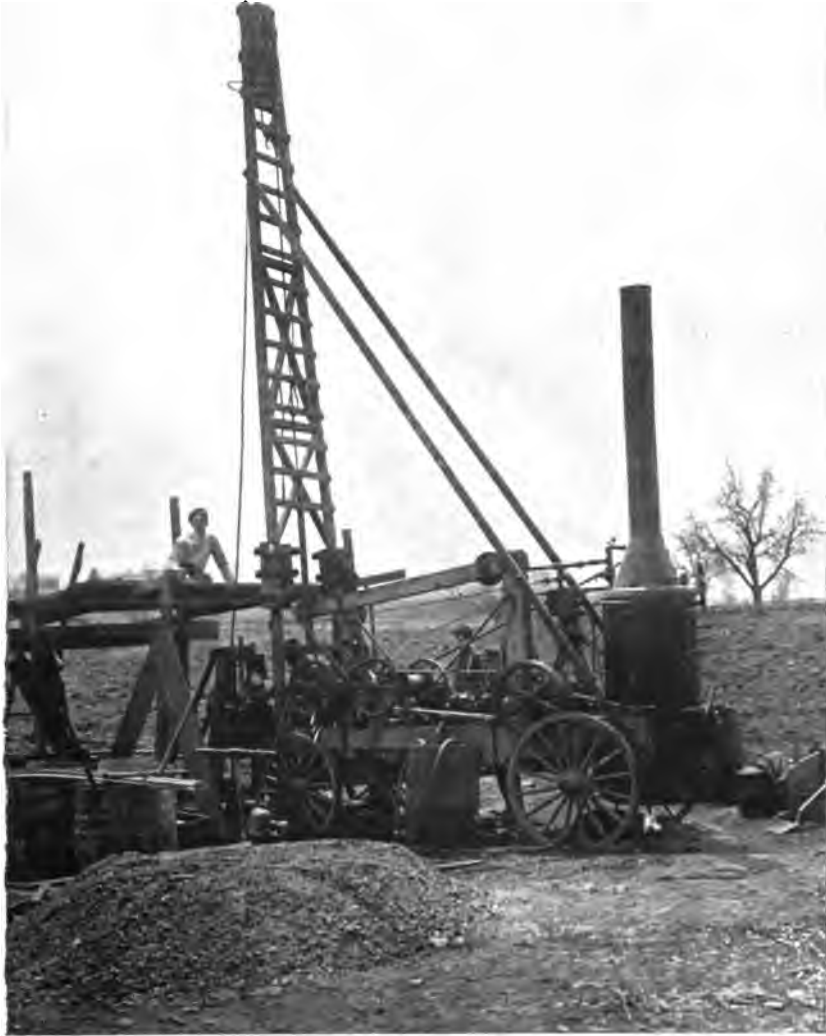
PLATE 19. —Board of Water Supply steam drilling rig. Machine operated as a "Wash Rig" to reach rock and then furnished steam for Badger-Sullivan diamond drill, raised and lowered drill rods, etc.
